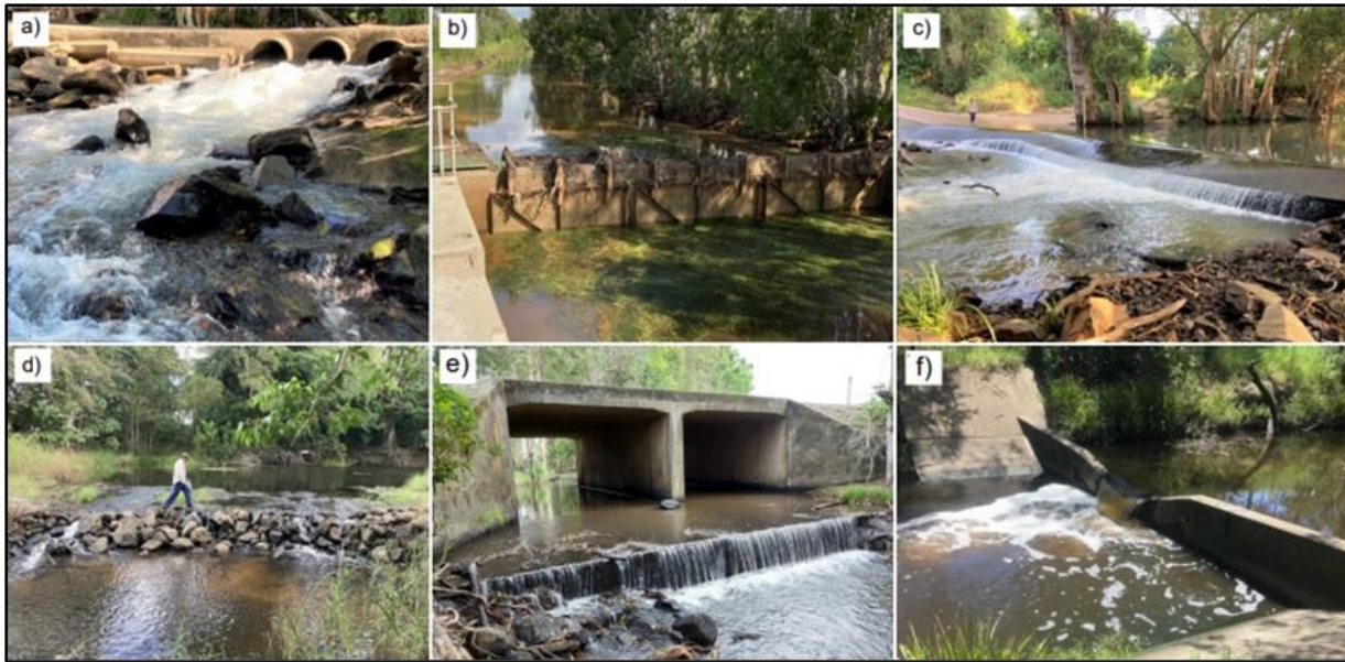
Figure 2: Barrier structures: a) pipe culvert causeway (Waterfall Creek), b) tidal floodgates (Mandam Creek) c) road causeway & apron drop (Frances Creek), d) rocky weir (Lagoon Creek), e) box culvert road crossing and concrete apron drop (Waterview Creek catchment), f) V-notch DNRME stream gauging weir (Warrill Creek).
