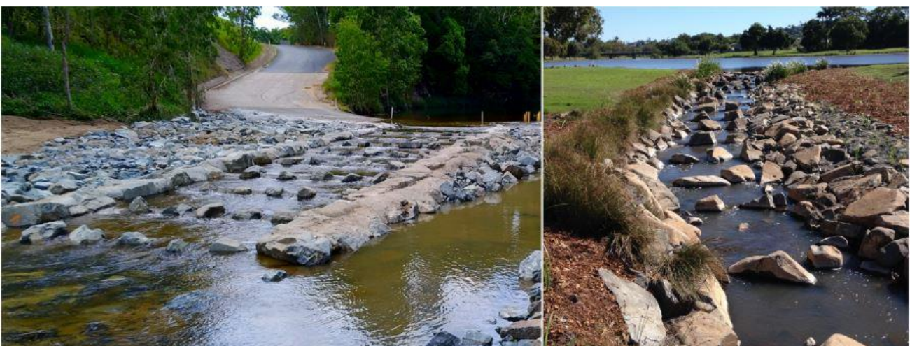
Figure 14. Showing rock ramp fishway constructed to remediate water surface drop barriers downstream from causeways; left Sandy Creek, Mackay (Palm Tree Road), and the Gooseponds (Janes Creek), Mackay City (right).
