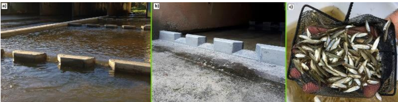
Figure 20. a) Retrofitted horizontal culvert baffles in operation under Paradise Road on Slacks Creek. Note: Nib wall to divert all base attraction flows down the fishway. Prior to remediating this barrier, the flow was spread out across four 2.4 m wide culvert barrels creating a shallow water surface barrier under base flow conditions. b) Horizontal baffles with the boxing recently removed c) Predominantly showing juvenile Sea Mullet and Striped Gudgeon captured successfully ascending through the horizontal culvert baffle fishway at catch rates of 256 and 793 individuals per day respectively.
