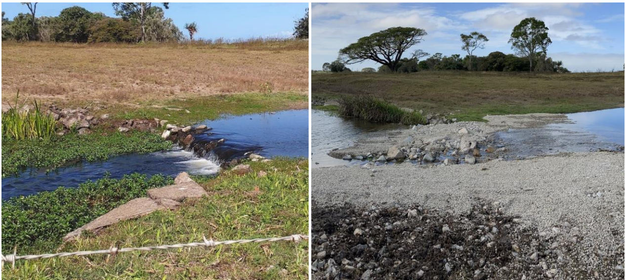
Figure 21. Left image: Pre-barrier remediation showing a bed-level crossing with a 300 mm vertical water surface drop on Palm Creek, Ingham. Right; Post-barrier remediation showing FFSP completed under the DAFs ADR. Note: Scour protection of various size rock (assist with interlocking) placed on a gentle gradient (1 high: 25 long), with a low flow channel. Larger rocks protruding from above the water level downstream from the crossing to reduce velocity and provide essential resting areas for migrating fish species.
