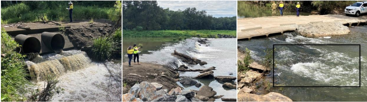
Figure 4: Left to right: Culvert causeway displaying high velocity flows through the pipes and two water surface drops; off the downstream extent of the pipe onto the apron, and from the apron to the waterway, showing a water surface drop barrier (centre) and showing a behavioural barrier due to insufficient light within the low-set culverts and velocity and turbulence (black polygon) barriers on the downstream extent of the structure due to a culvert aperture <40% of stream width (Coomera River, SEQ).
