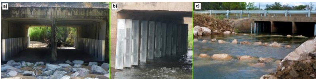
Figure 19. a) Vertical culvert baffles with scour protection (Aims Rd, Townsville) b) Close up view of vertical baffles retrofitted to a culvert c) Vertical baffles in conjunction with a rock-ramp fishway (Sheepstation Creek, Ayr).
