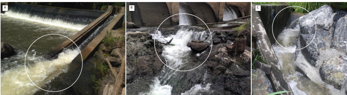
Figure 3: Showing northern hemisphere 'salmonid' style fishway designs exhibiting hydraulic conditions in excess of the swimming abilities of most native freshwater fish species. a) Denil fishway located on Luscombe Weir (Albert River, Queensland) showing steep gradient and excessive velocities (note baffles removed). b) Showing the bottom section of the Mt Crosby weir pool and weir fishway (Brisbane River). Note the inadequate fishway entrance with excessive turbulence associated with the large water surface
