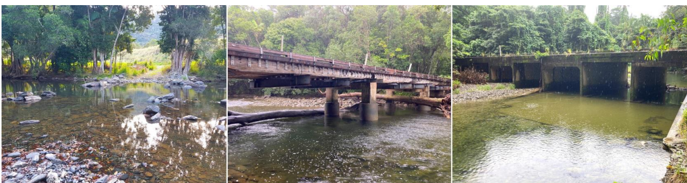
Figure 10. Typical non-fish barriers validated during ground-truthing. From left to right; Natural bed level crossing (Mowbray River), Bridge (Noah Creek), and a box culvert causeway encompassing the full stream width and constructed below bed level (Cooper Creek).
